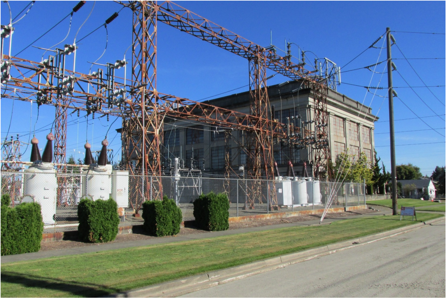
Figure 19 Cushman Substation view southeast
