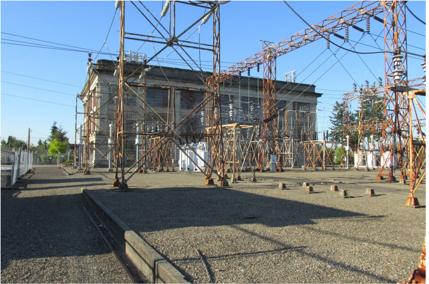
Figure 20 Cushman Substation view south
